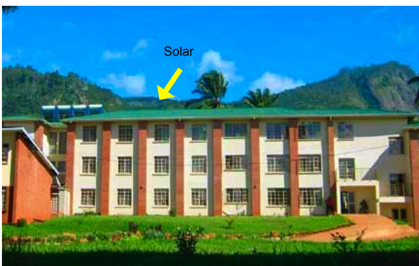
Figure 2: Solar geysers installed on student hostels at Chancellor College, Zomba
