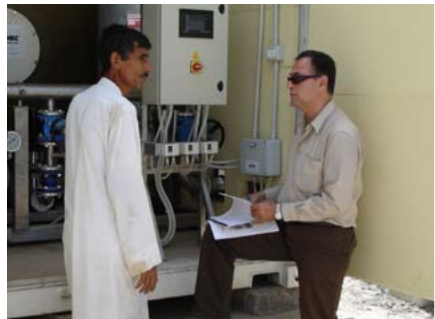
The water plant facility at Al-Masahab
