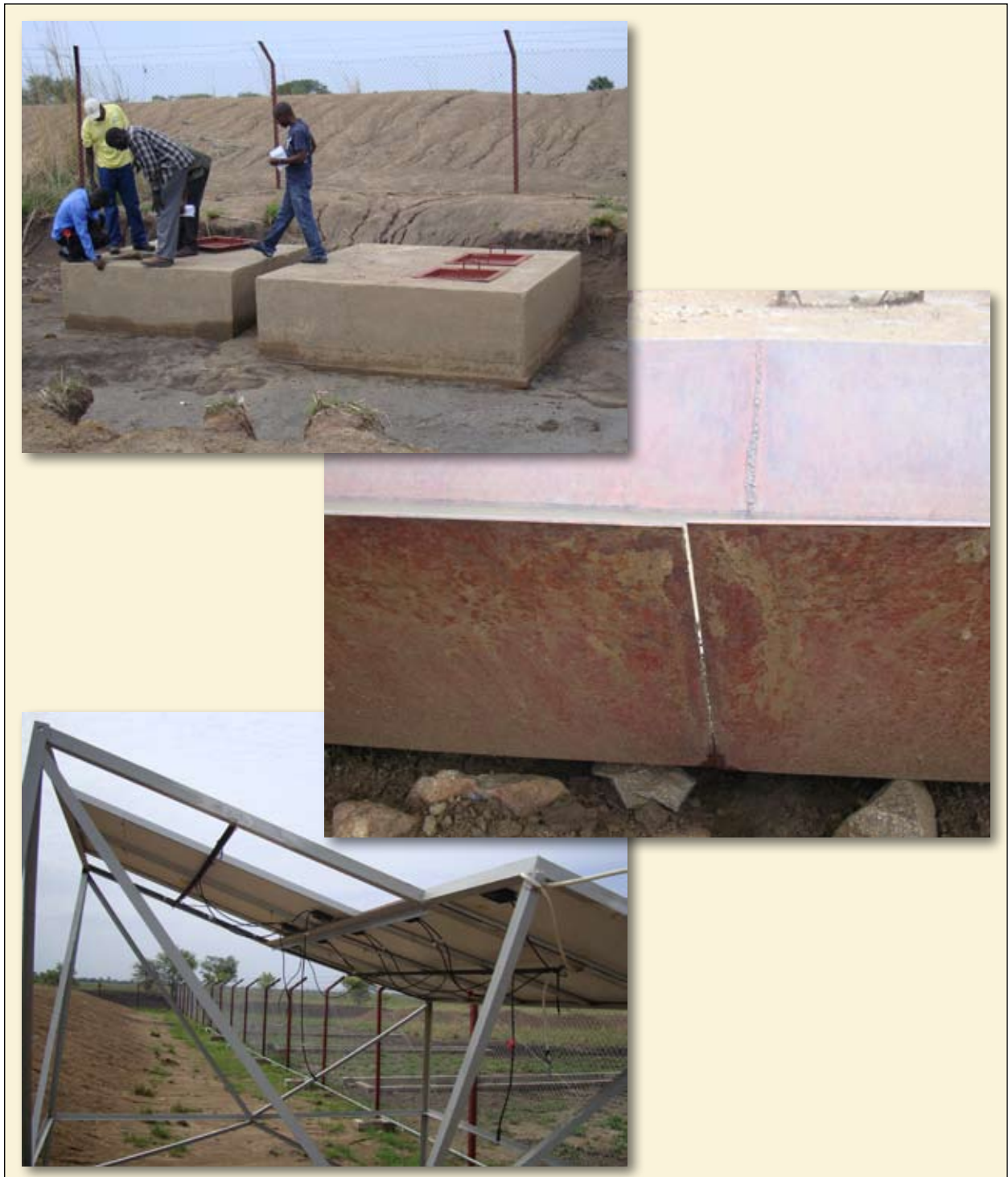
Figure 2. Wrongly set intake box (top); Poorly welded cattle trough (middle); Poorly fixed solar panels (bottom)
