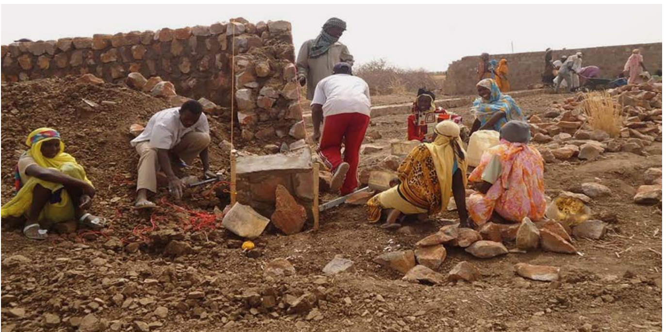
Community members volunteered to rehabilitate the Eware water retention structure
