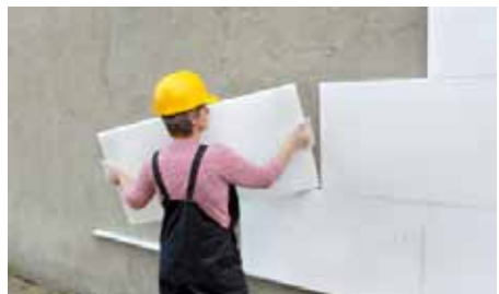
Figure 25. Wall foam insulation to save heating energy
