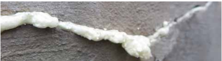
Figure 34. Foam wall crack
