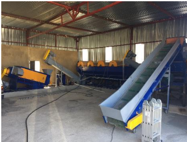
Plastic Wash Plant
