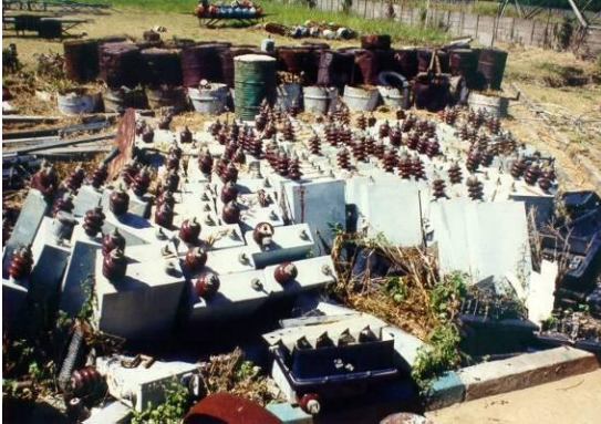
Picture 84: Bad example I (open air storage)
