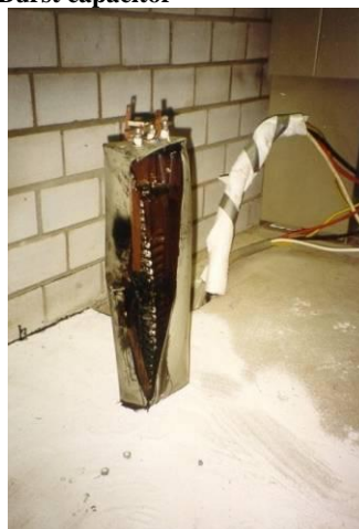
Picture 50: Burst capacitor
