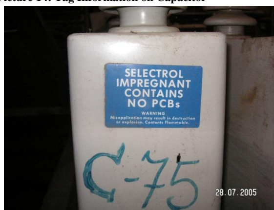
Picture 14: Tag Information on Capacitor
