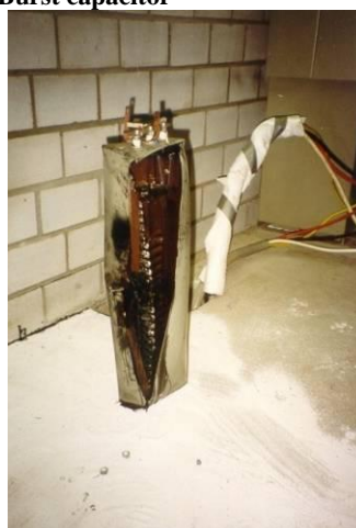
Picture 50: Burst capacitor
