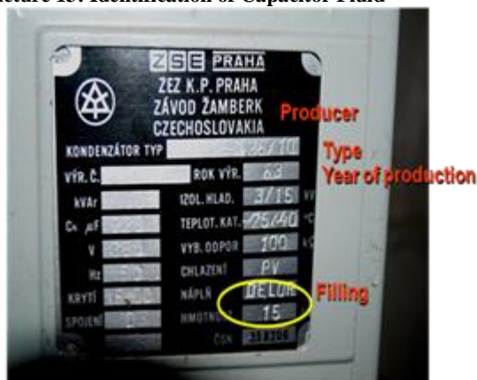
Picture 13: Identification of Capacitor Fluid
