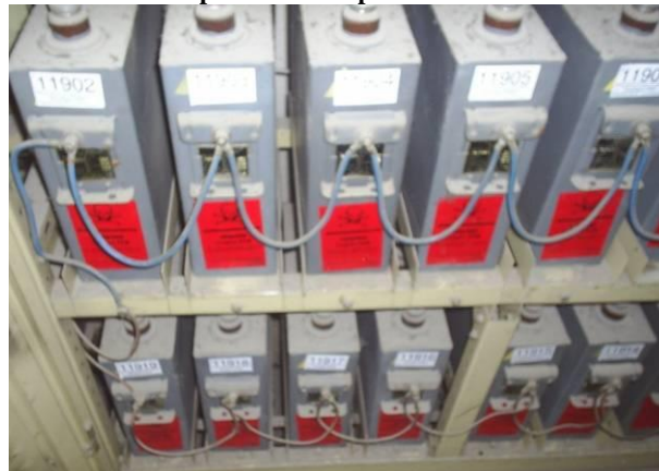
Picture 36: Example labelled capacitors
