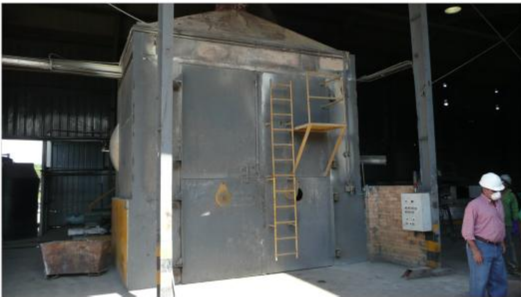
Fig. 27: Furnace of Industrias Meteoro S.A. - Dominican Republic [25].
