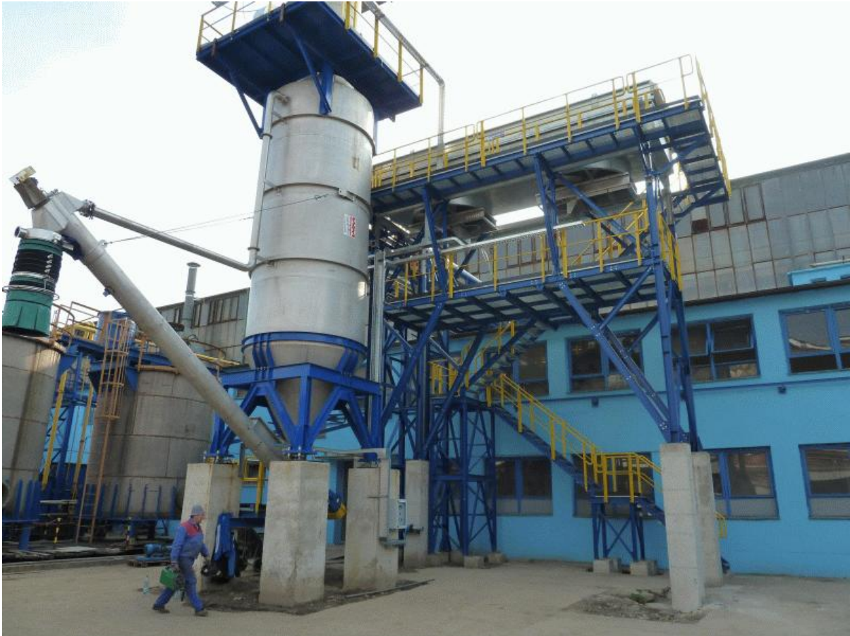
Fig. 19: Secondary lead installation of the company Mach Trade (Slovakia)
