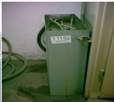
Picture 56: Inventoried and labelled capacitor
