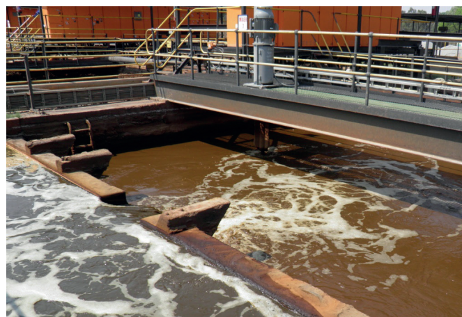
Mine water treatment facility, West Rand, South Africa Credit: Tamiru Abiye
