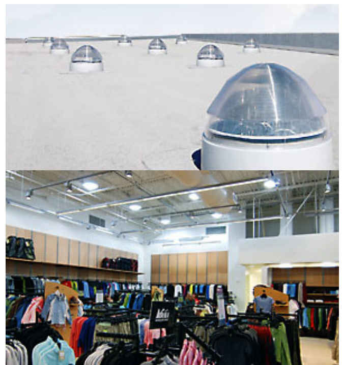
Figure 34: Solar tubes conduct daylight into a room
