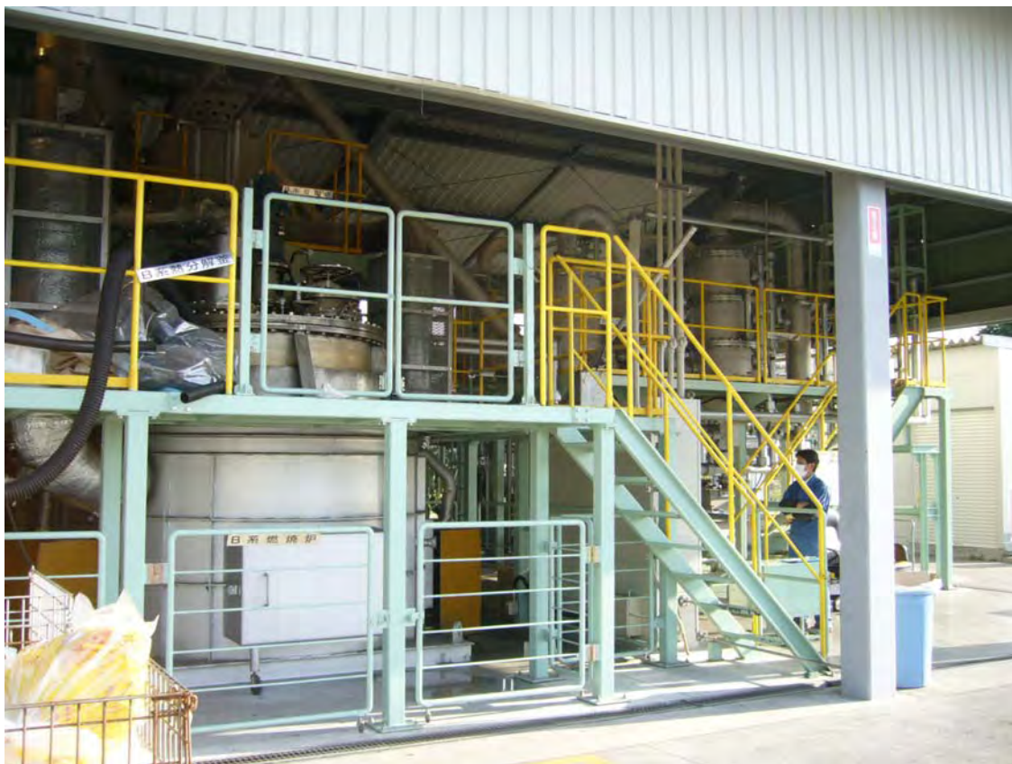
Figure 8.1: Fuel Oil Production Plant at a packaging manufacturer in Gunma Prefecture.
