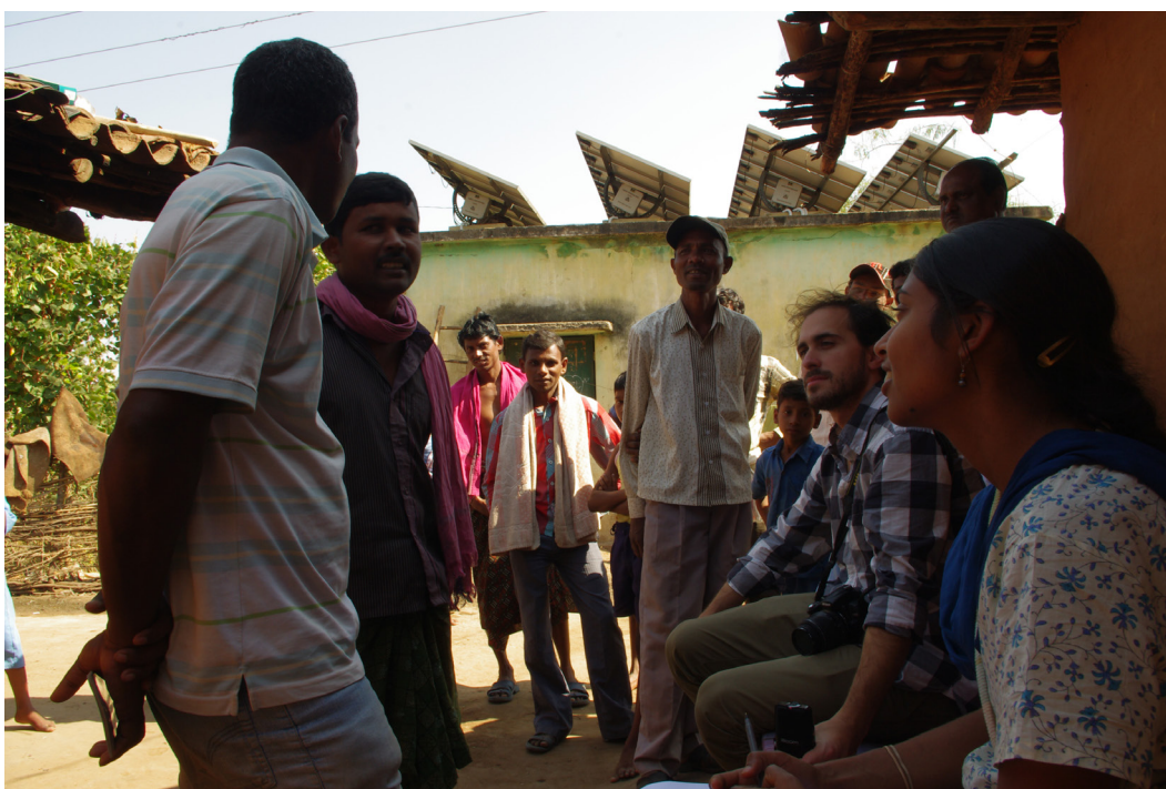
A community meeting to discuss the village's 2 kW PV system in Orissa, India
