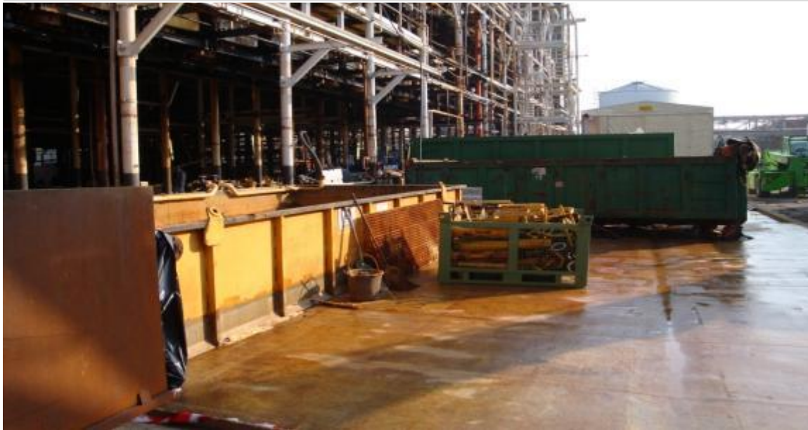
Working area for safe handling of contaminated equipment connected to the Hg effluent treatment unit, regularly washed down with water
