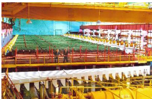
Mercury-cell chlor-alkali plant
