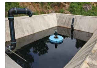
Figure 8: Leachate treatment plant, La Digue, July 2018
