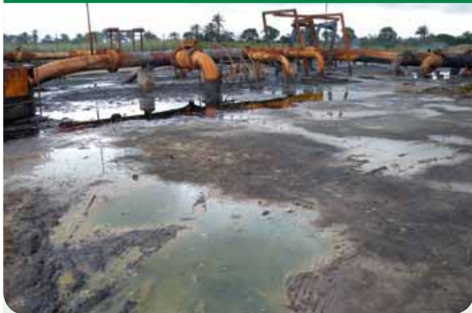
Oil contamination at the Bomu flow station in K-Dere, Ogoniland, Nigeria. Credit: UNEP
