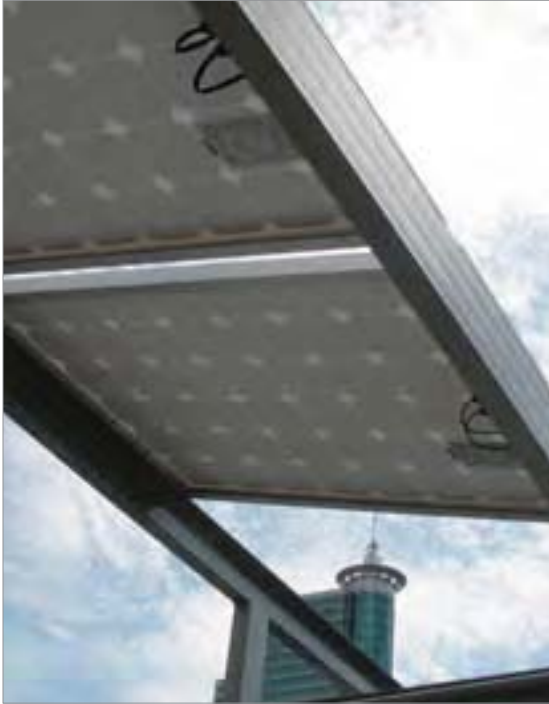
Solar panels on the roof of the new car parking building at ADB headquarters
