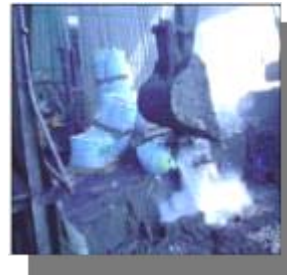
Waste Treatment Plant
