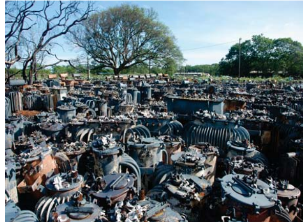
PCB-containing equipment after a fire accident (Joint UNEP/OCHA Environment Unit, field visit of the interagency team, 2015)
