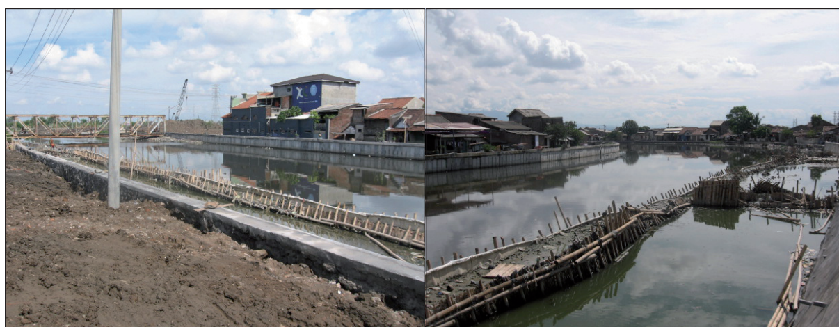
Figures 4. and 5. Early construction phase of the Banger Polder Pilot System (2011) Photo credits: Dana Adisukma
