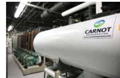
Fig. 2 Photos of the transcritical CO 2 system at Sobeys designed by Carnot Refrigeration.
