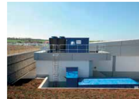
Fig. 2 Photo of Outdoor Integral Chiller Plant Installation
