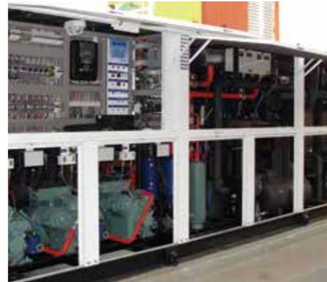
Fig. 5 The refrigeration system
