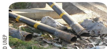
Figure 27: Detail of the weak anchor and hollowness of bollard.
