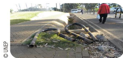
Figure 26: Broken bollards on UN Avenue due to a traffic accident.
