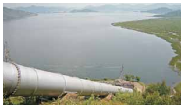
Almost half of Rwanda's electricity supply is derived from hydropower, which potentially may be compromised by erratic rainfall. Shown here is the Ntaruka hydropower plant in the Northern Province
