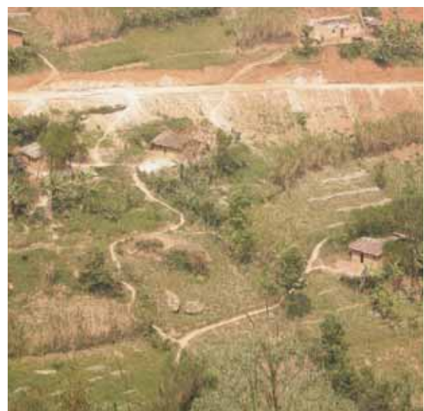
Secondary unsurfaced roads were observed to be important hotspots of soil erosion
