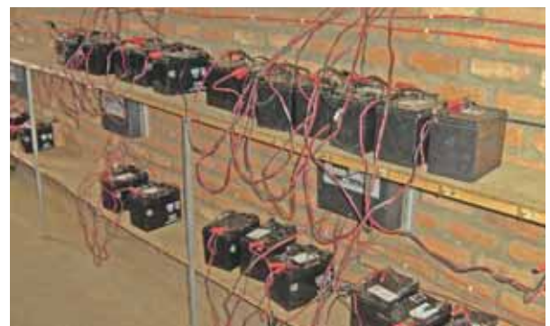
Solar battery charging at Arusha imidugudu in Gishwati
