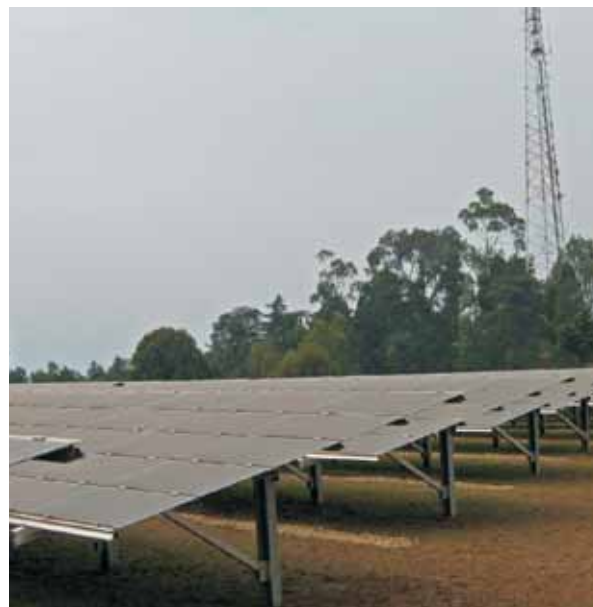
The solar power plant at Jali Hill in Gasabo District is one of the largest in Africa
