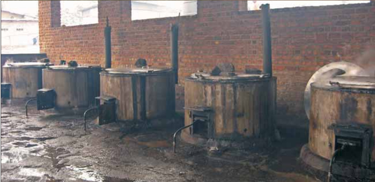
Biogas from underground digesters is piped to the Remera prison kitchen. Large-scale biogas plants have proven an effective means in dealing with the sanitation and fuelwood problems created by the sharp rise in Rwanda's prison population following the 1994 events
