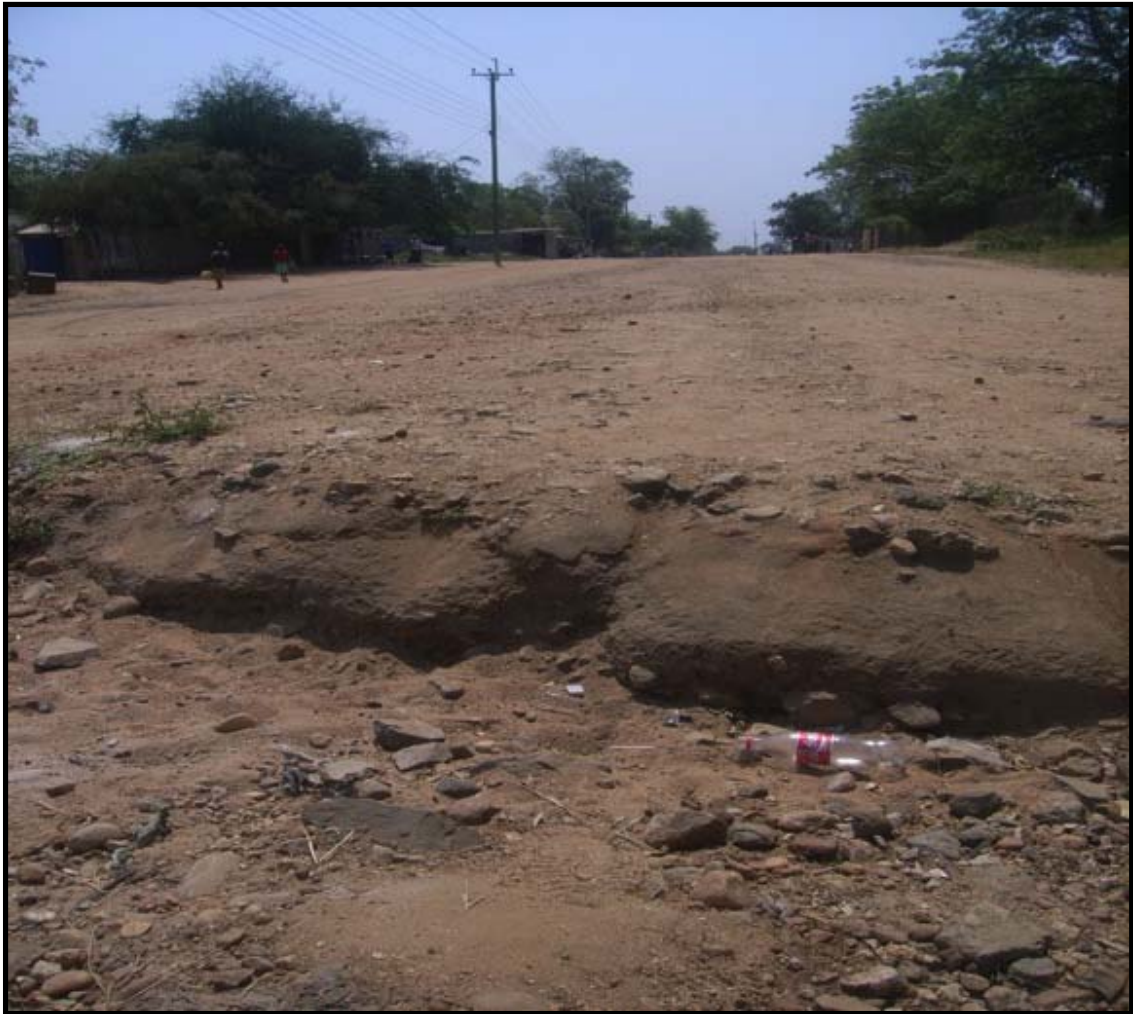
Road conditions such as these in Juba are having a serious impact upon waste collection vehicles, in particular the new compactors which carry a far higher pay-load
