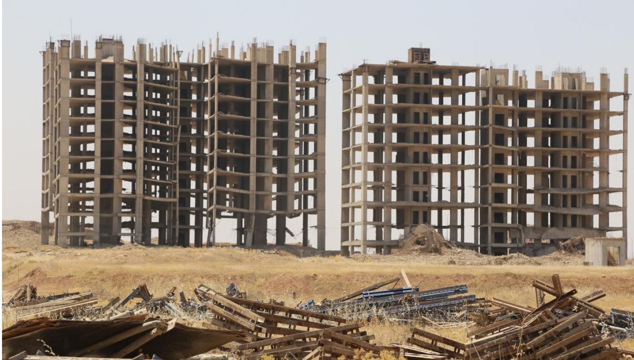
The foundational pillars of these buildings were blown-up by ISIL, necessitating their demolition © UN Environment
