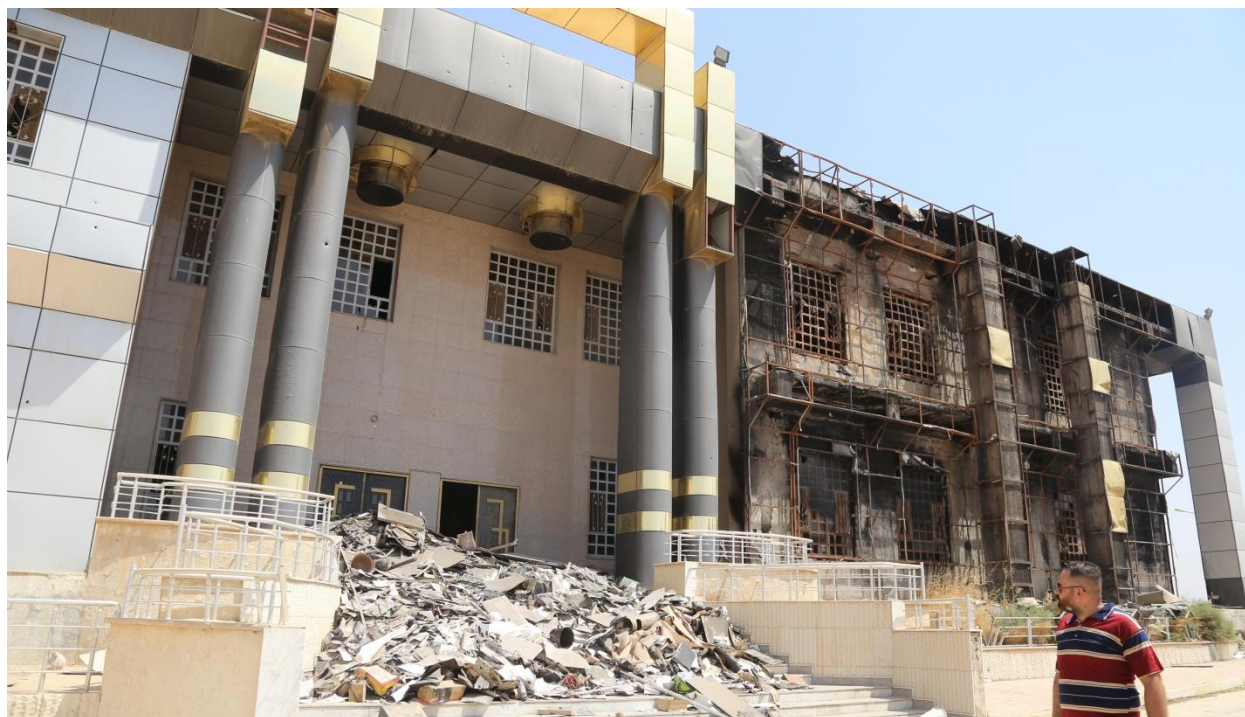
Mosul University's Environmental College was ransacked by ISIL who used it as one of their command centres © UN Environment
