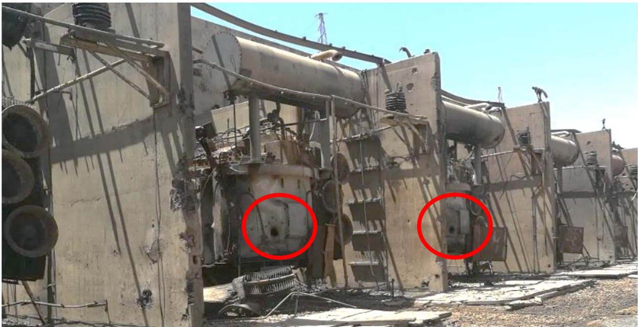
At Western Mosul's main power station, heavy calibre rounds were deliberately fired into a block of power transformers filling the basement of the building below with up to 3 metres of potentially toxic transformer oil © UNDP
