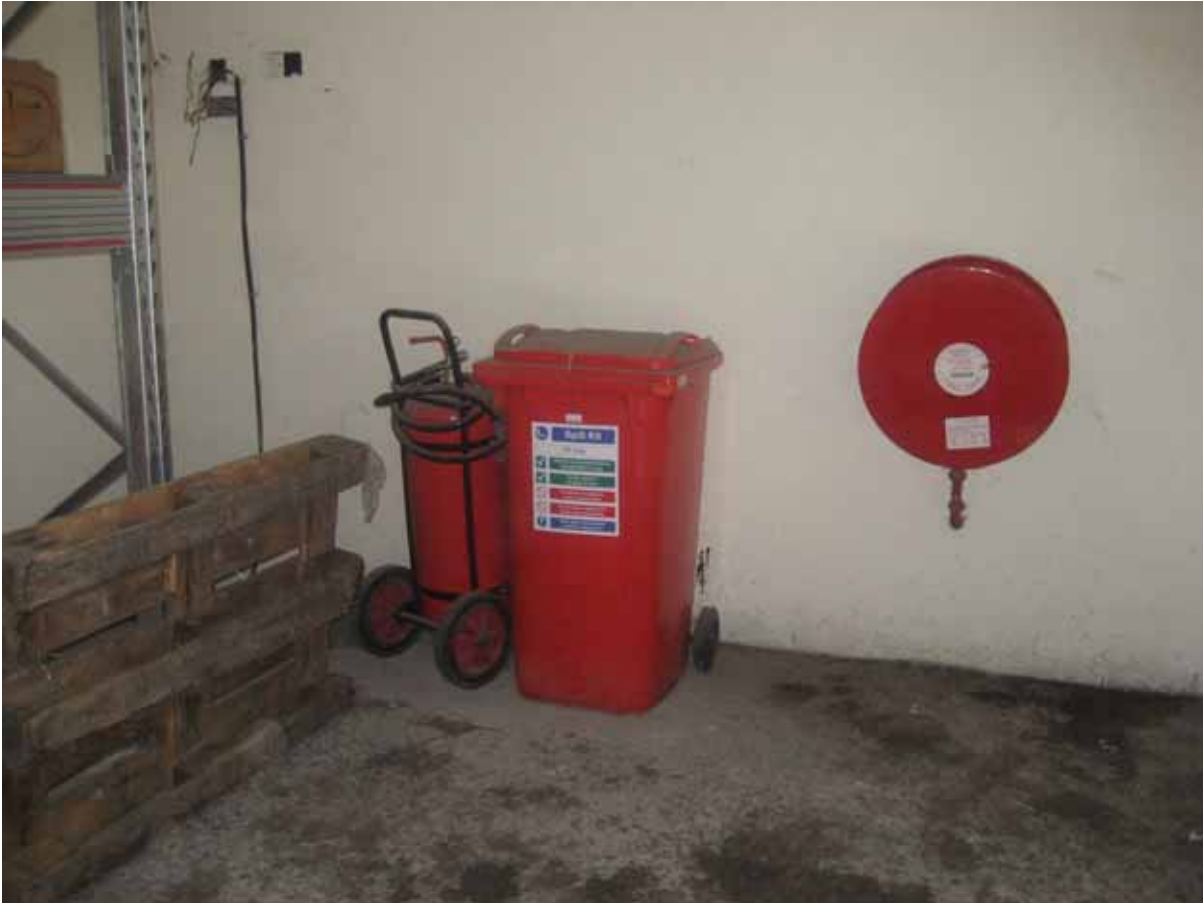
Figure 3: Fire fighting equipment is strategically placed within the base
