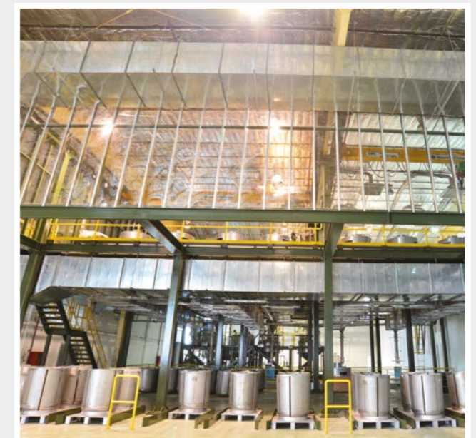
Mercury waste treatment facility at BMT Pacific Co. Ltd © BMT Pacific Co. Ltd.
