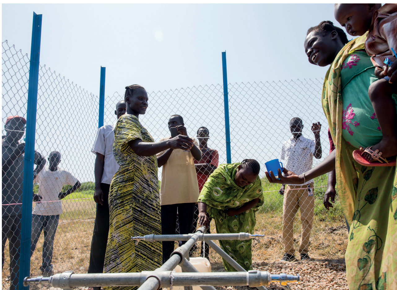
Solar powered mini water-yard facility in Gormoyok Village in Juba County, Central Equatoria State. Photo credit: UN Photo/JC McIlwaine
