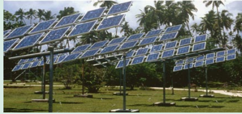
Figure 12.5 Solar panels on Nukubati Island
