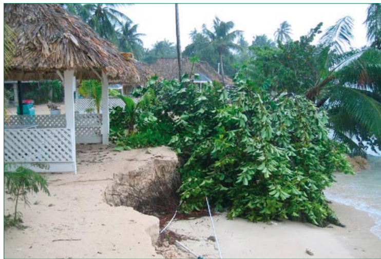
Figure 9.4 Erosion of shoreline and damage to tourism infrastructure due to hurricane Ivan in Tobago
