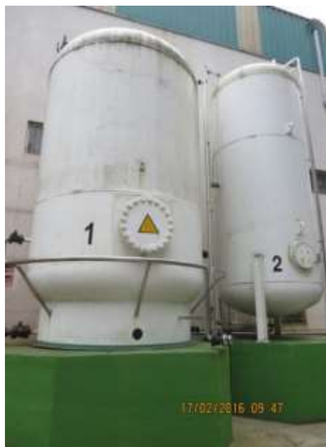
Storage facility R22 (37,000 kg)
