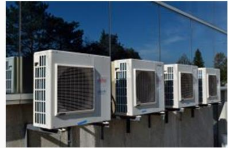
The rising global demand for air conditioning and refrigeration helped push through an amendment to the Montreal Protocol that will limit the use of hydrofluorocarbon refrigerants.
