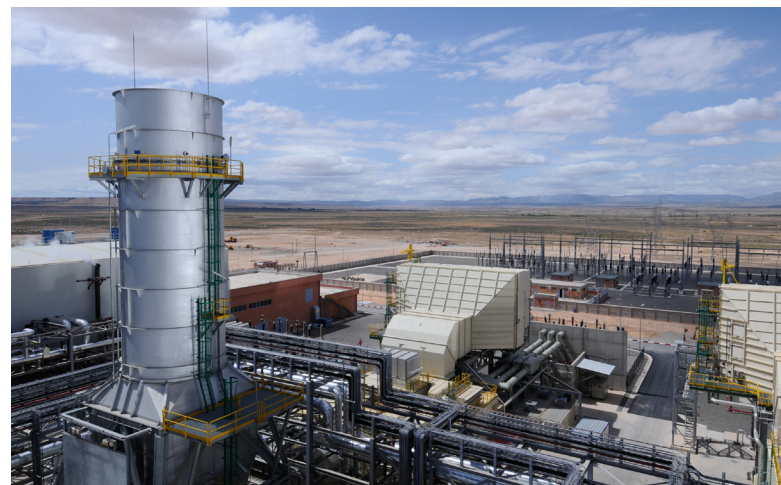
Thermo-solar power plant in Morocco (World Bank 2010)
