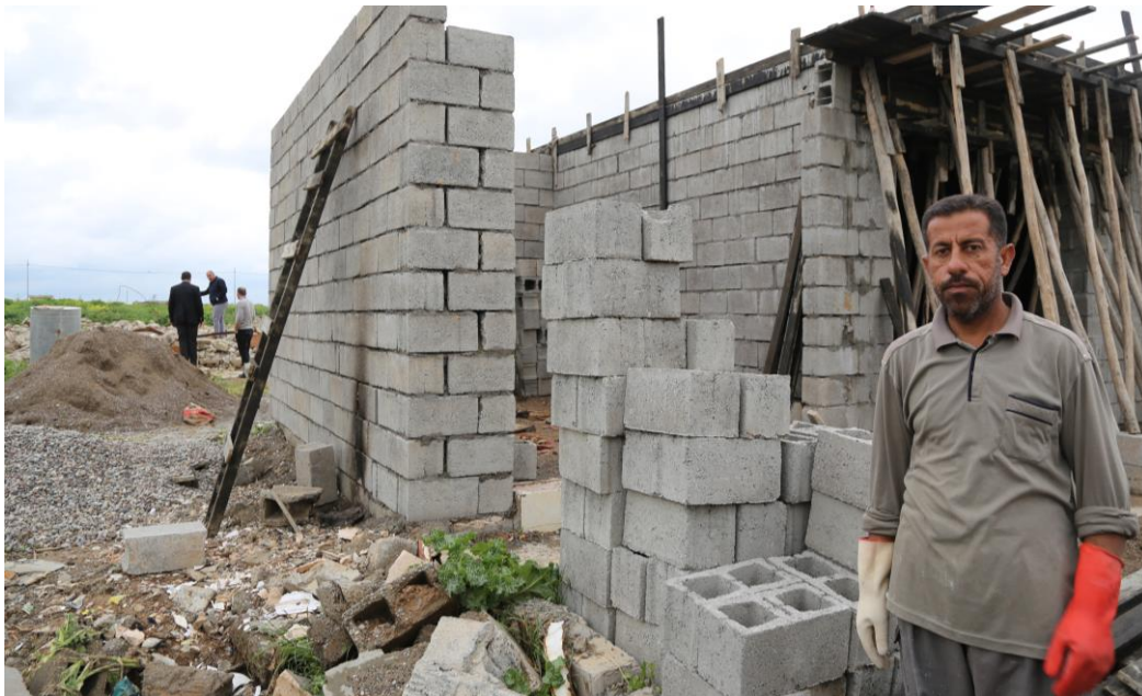
Photo 3: Very few homeowners are returning to rebuild their houses, largely due to presence of debris hindering access and the lack of basic services (water & electricity).
