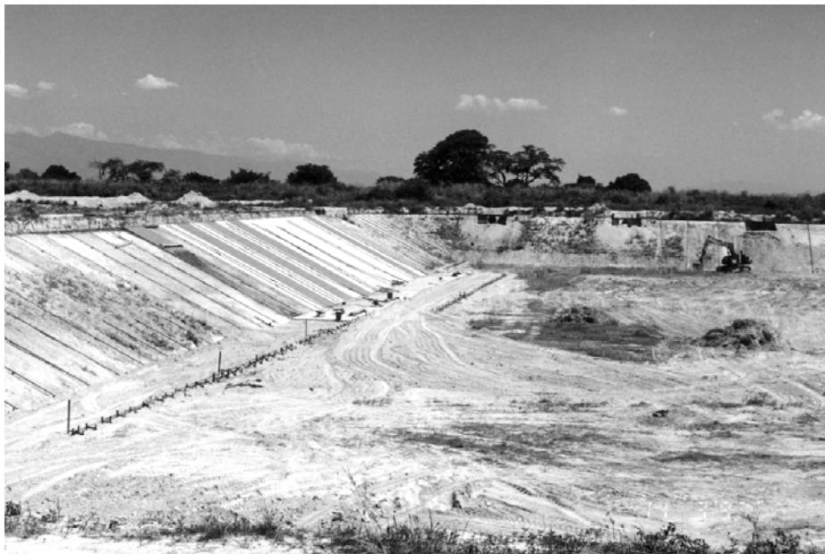
Construction of concrete liner on the side slopes of the primary treatment cells at the Los Guayos treatment plant.
