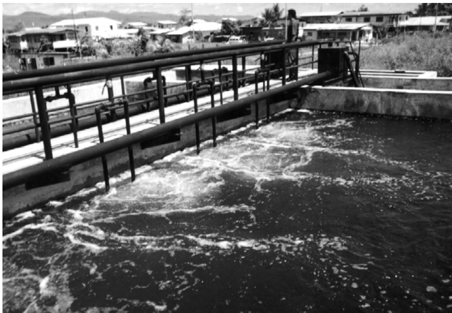
Aeration tank at the small extended aeration plant in Charleyville.
