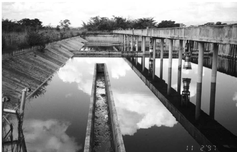
MSBR tanks at the Mariposa treatment plant will use high-speed direct-drive propeller aerators suspended from concrete access bridges.
