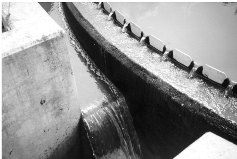
Effluent from the secondary sedimentation tanks at the Arima sewage treatment works.
