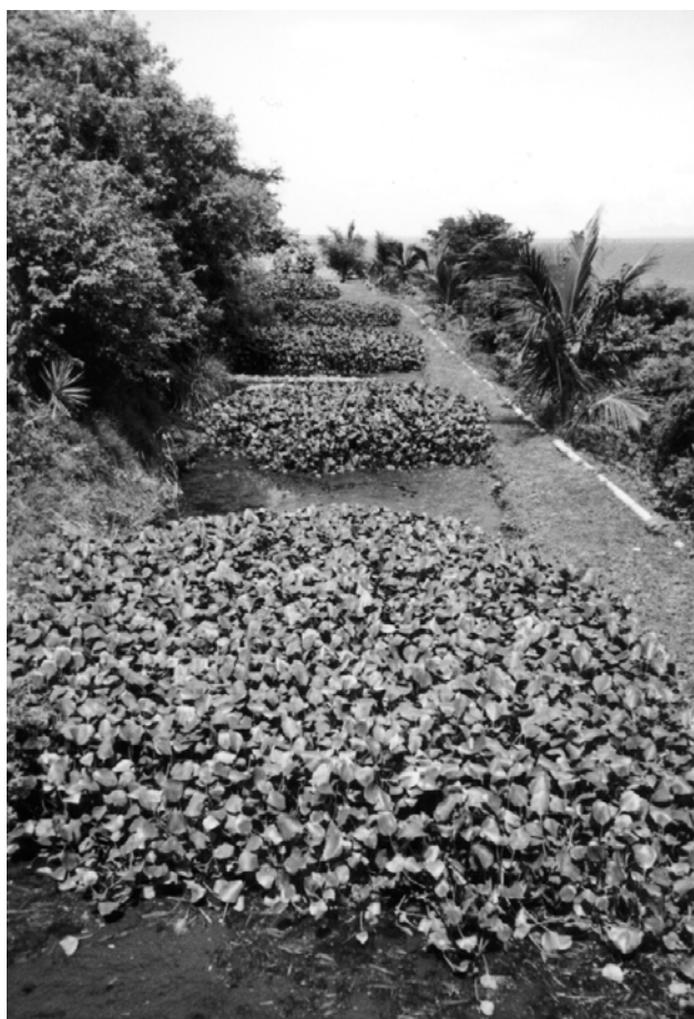
Constructed wetlands in a package treatment plant serving a hotel in St. Lucia.
