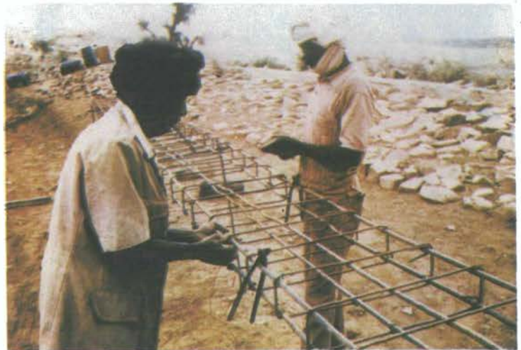
Men constructing internal steel reinforcement for a small dam in Mauritania. (UNSO/UNEP)
