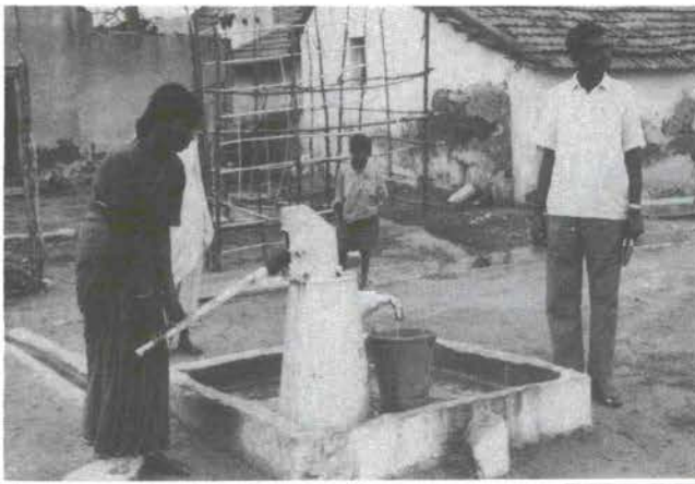
This pump handle is too low for operating comfort
