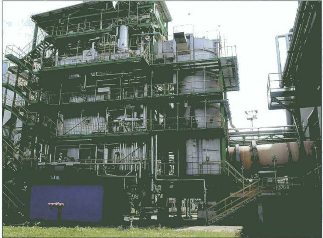
Waste incineration plant for termic destruction of substances CFCs and HCFCs in Ostrava ▲►
