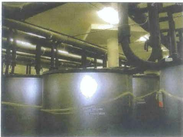
The cooling facility in Szuka Arena
