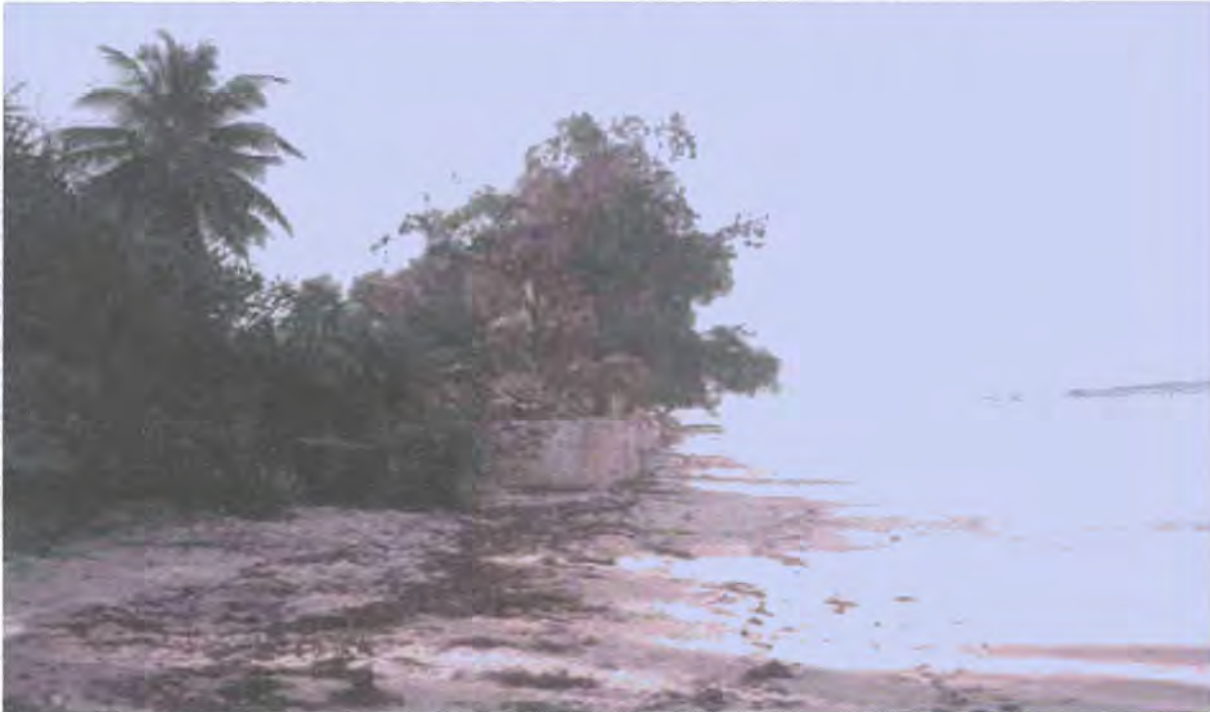
Plate 1.2. A concrete barrier constructed to protect beach infrastructures against heavy storms. Its long-term impact might be even more disastrous (Photo by Dalmas, July 2000)
