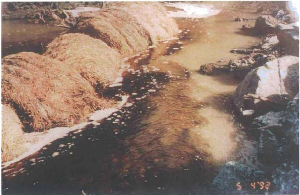
Picture 12 : The use of bales of hay for water management. Used here as a diversion.
