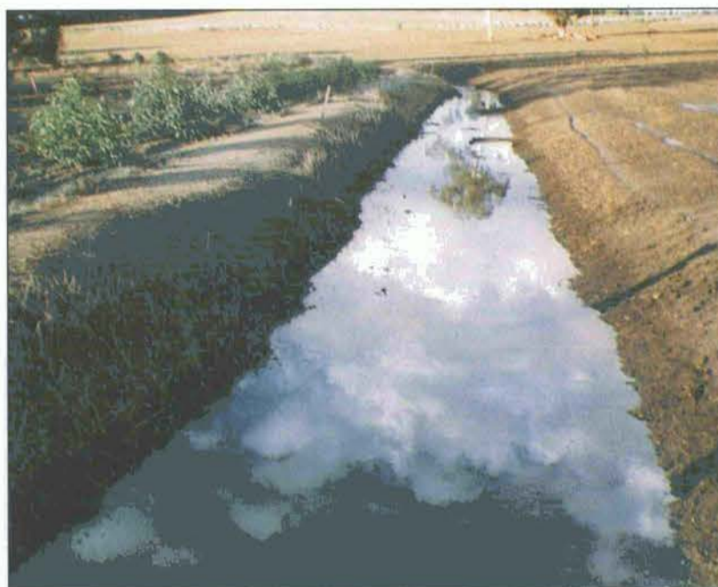
Figure 4.52 A newly dug interceptor drain. On the left is the bank formed of the excavated soil, on which the first plantings for the windbreak can be seen
