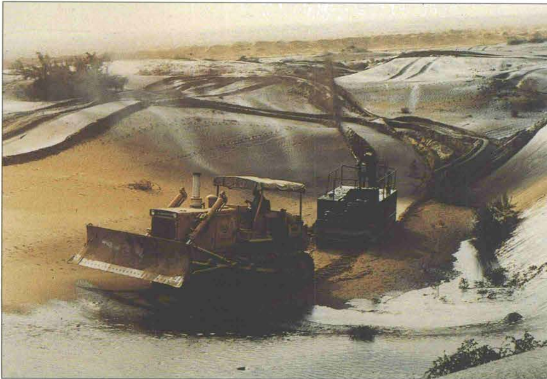
Figure 1.18 Stabilisation of mobile sand dunes, as here in Iran, can be achieved by methods including spraying with oil, tar or synthetic materials (UNEP/SA Rizehkar/Topham)
