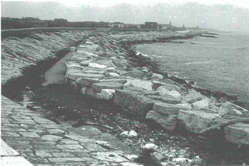
Figure 69 Sea level rise resulting largely from land subsidence in the Venice region has led to beach erosion on the enclosing barrier islands. Here at Litorale di Pellestrina the lost beach has been replaced by a sea wall and boulder rampart
