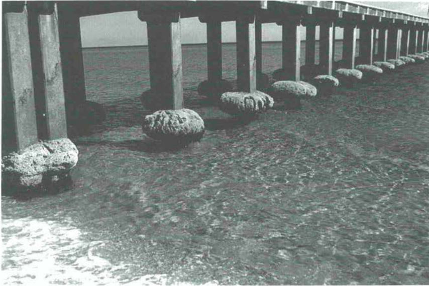
Figure 20 Cushions of Galeolaria caespitosa on pier supports at Rosebud, on the shores of Port Phillip Bay. The upper limit of these cushions is likely to be raised in response to a rising sea level
