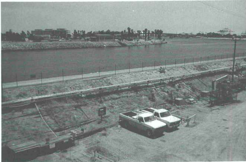
Figure 59 Riverside walls keep the sea out of the subsided dock area west of Long Beach, California. Note the active oil well to the right of the parked cars
