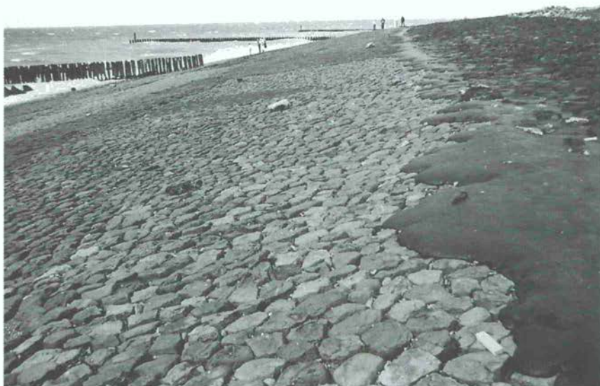
Figure 68 The seaward slope of the sea wall at Westkapelle forms a stable, but artificial, coastline. Wooden posts form rough groynes, intended to trap sand and form a beach, but there is very little beach material here
