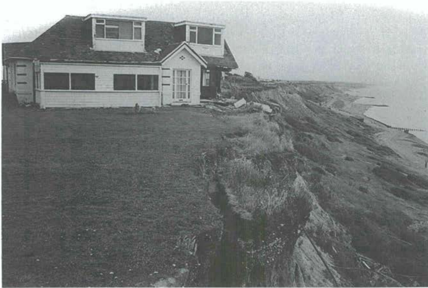
Figure 79 Cliff recession has forced the abandonment of this house on the coast of Christchurch Bay, southern England
