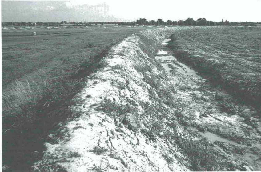
Figure 40 An earth embankment built at the rear of a salt marsh near Bosham, southern England, to prevent marine submergence of farmland (right). As sea level rises, such an embankment will prevent the landward migration of salt marsh indicated in Fig. 41
