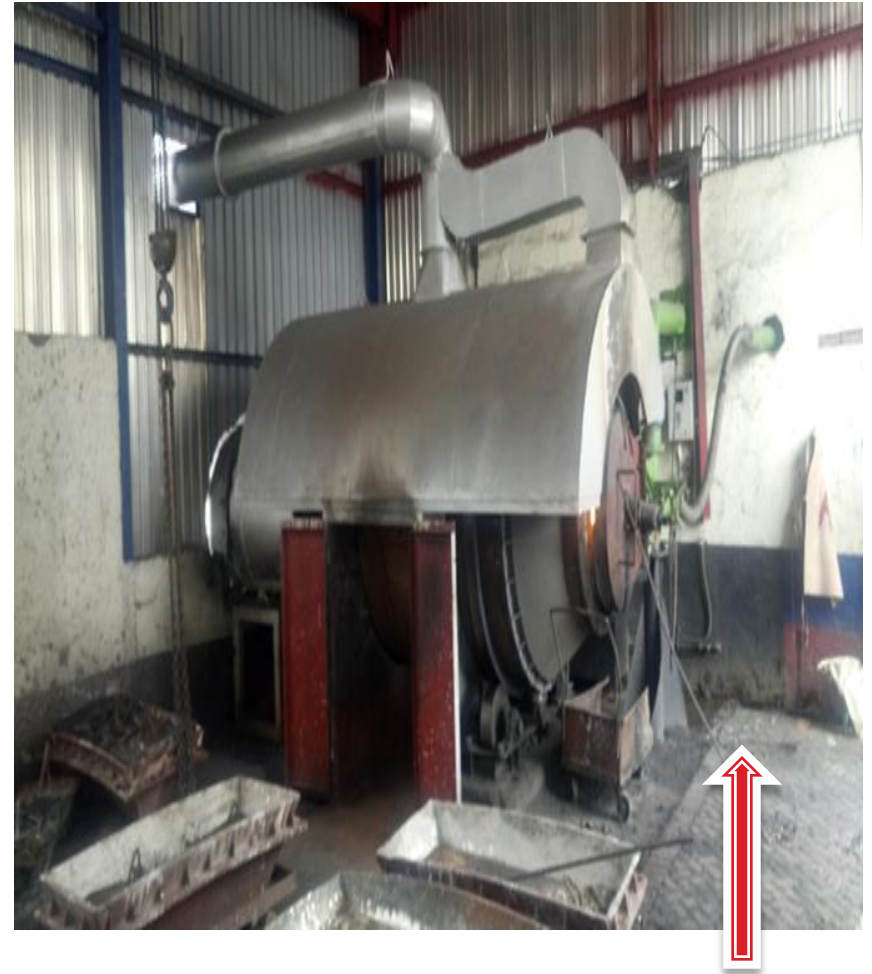
Upgraded extraction system
