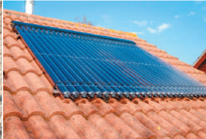
FIGURE 4.16 Rooftop solar water heaters/solar thermal collectors (YouGen United Kingdom)
