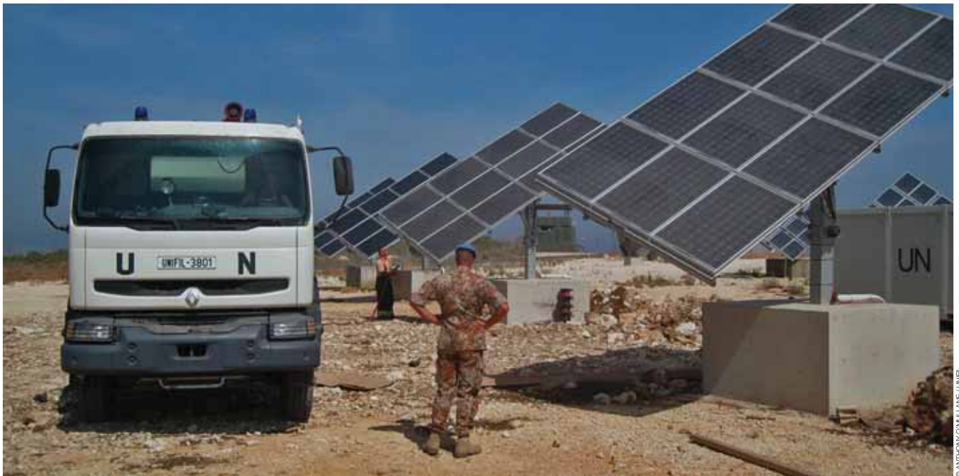
The United Nations Interim Force in Lebanon (UNIFIL) uses solar panels to increase energy efficiency
