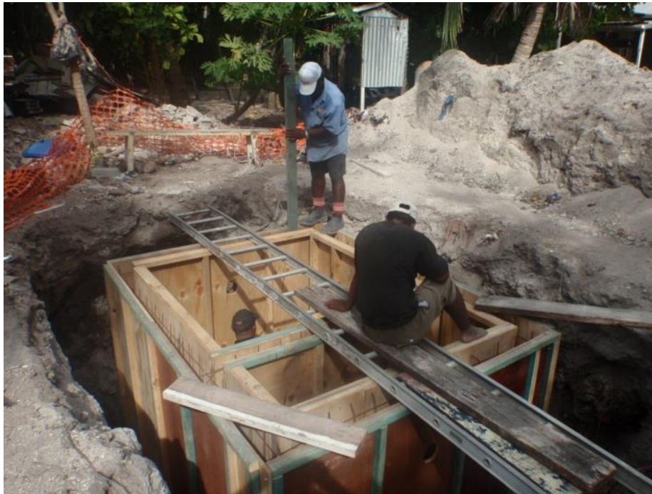
(Contractor positioning the conventional Septic Tank mold at the demonstration community in Ewa. 22/02/2011)
