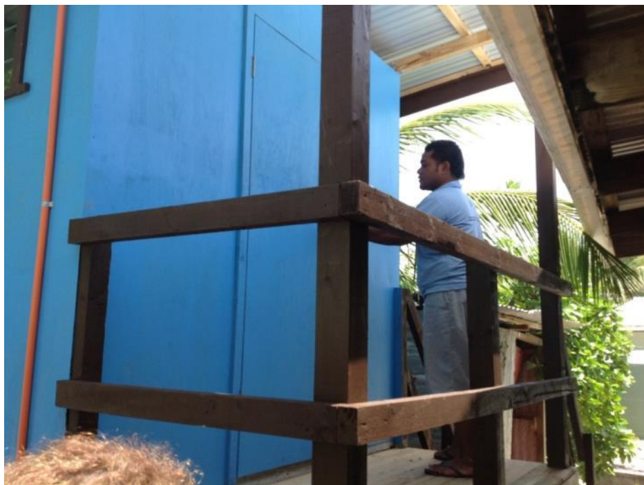
(Pisi Seleganiu inspecting one of about 50 compost toilets developed and installed in Tuvalu under the IWRM Project)
