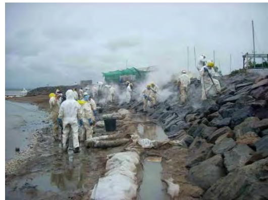
Example of high pressure washing with oily water recovery downstream in pits with sorbent, Loire estuary (France) 2008 Photo: CEDRE
