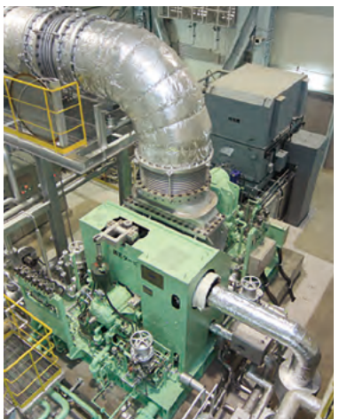
(b) Turbine generator
