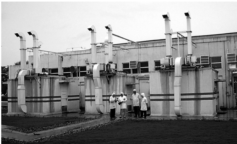
These outside gashouses were constructed by an aerosol filler to the specifications indicated in this manual.
