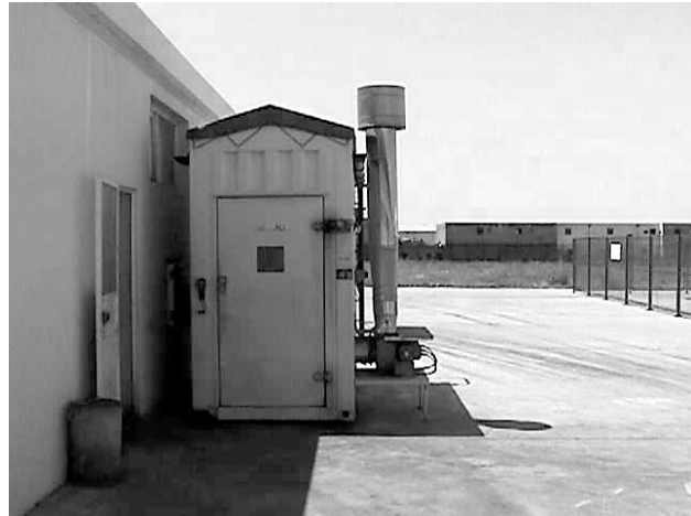
This small gassing room in Tunisia has only one exhaust stack, but two speed extraction.
