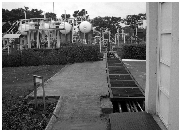
This excellent installation in Thailand shows protection posts, good fencing, and a parallel unloading. Note the height of the "pipe bridge."
