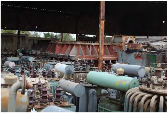
View of transformers stored at the site
