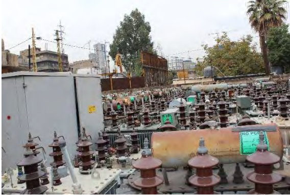
Transformers stored in the open, exposed to weather conditions
