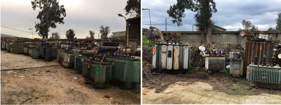
Figure C-4: Storage area for contaminated transformers
