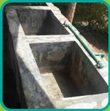
Cleaning bay with fitted taps
